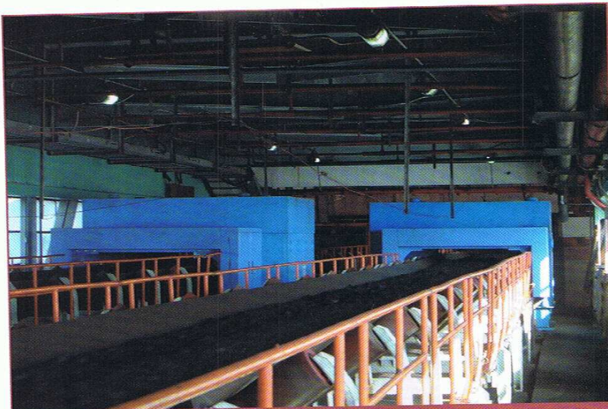
Twin Coal CNA in a Chinese power plant for boiler combustion optimisation.
