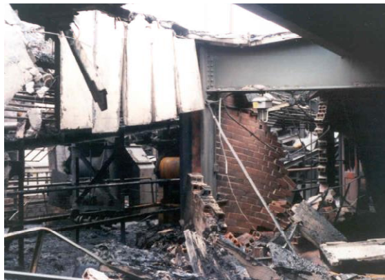
Figure 3. Tripper room after explosion at WPS J. P. Pulliam Generating Station
